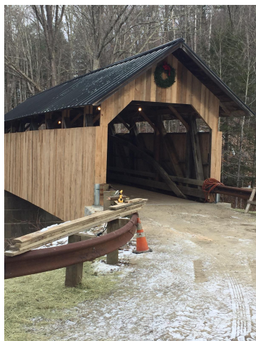
News from VT Digger, January 23, 2017 and Melrose Duff. Photo Courtesy Vermont Agency of Transportation)
