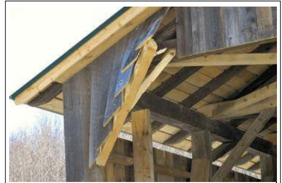
Canyon Bridge Damaged [WGN45-08-01] Photo by John Borthwick Feb 5, 2005
