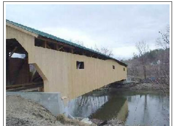
Poland Bridge - On upstream side looking north. Windows cut, siding following the top of the arch.
