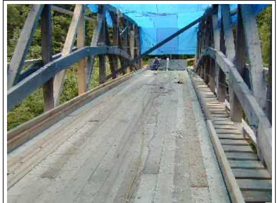
The transverse sub-floor planks have been placed and spaced. The longitudinal deck planks are being lag bolted to the sub-floor. Photo by Joe Nelson, August 23, 2004
