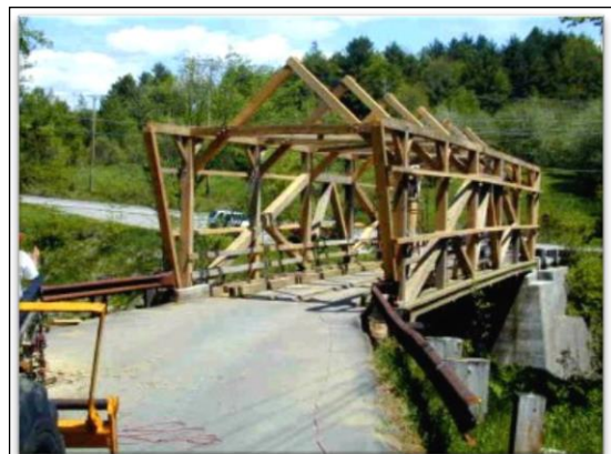
Power House Bridge Coming along nicely, thank you! Photo by Joe Nelson, May 28, 2002
