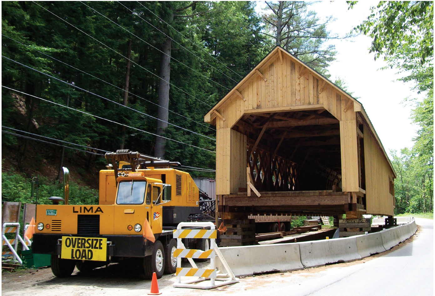
The final stages of construction of the new covered bridge took place in the roadway near the job site, just prior to demolition of the old bridge and the salvage of its materials for recycling.
