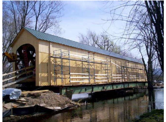
Salisbury Station Bridge, Good for the next 100 years photo by Joe Nelson, April 23, 2008
