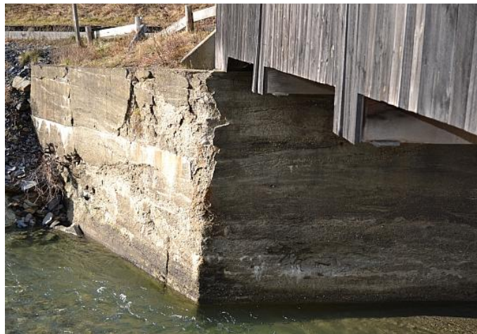
The West Abutment is in poor condition
