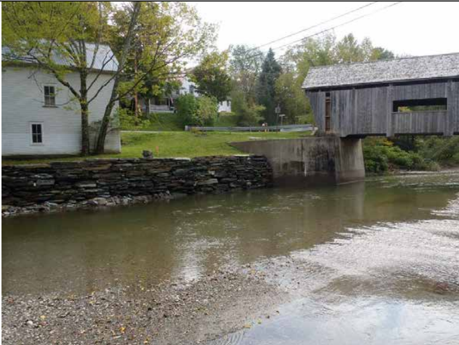
Mad River - Covered Bridge looking upstream at laid-up stone wall, east side of the stream.
