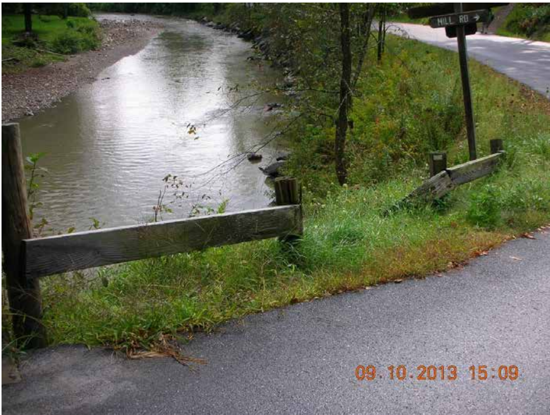
Photograph 10 - Substandard and Damaged Approach Rail at SW corner
